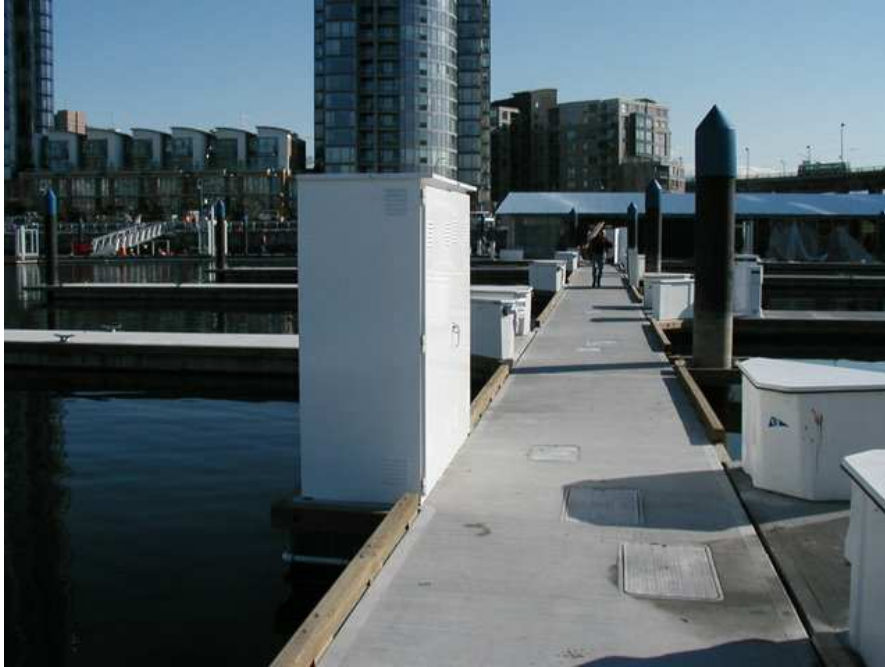
Concrete Dock with Built-in Utilities
